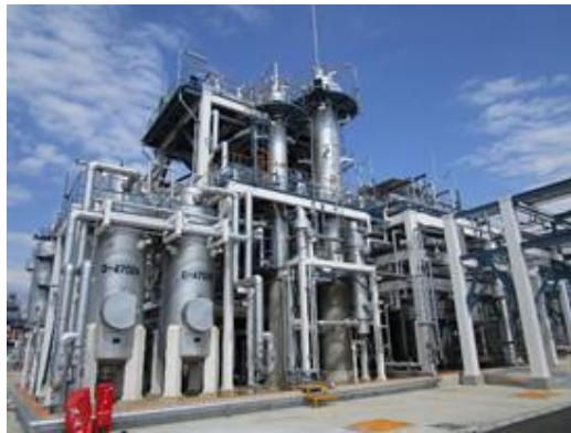
New LUCANT™ Plant at Ichihara Works
